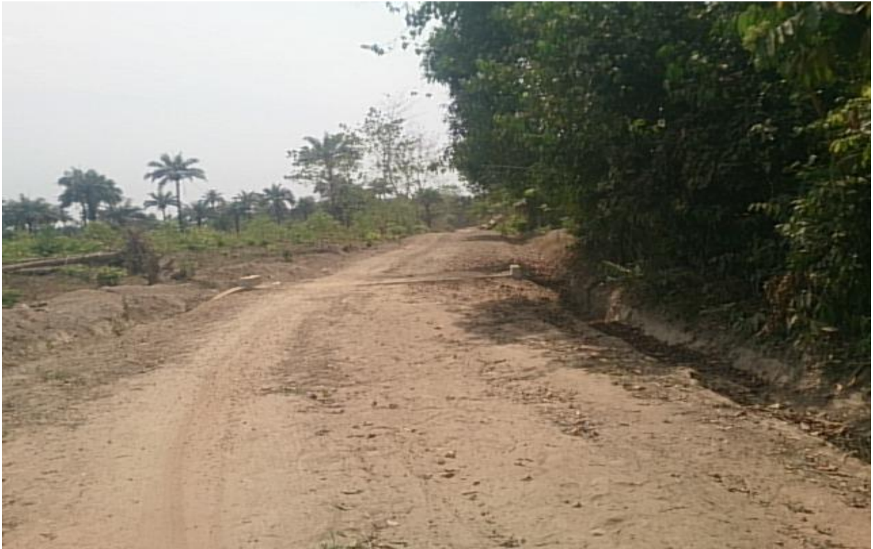
Road Constructed by Miro Forestry SL Ltd leading to Manjehun, Patfumayagbo, Mabilla Banna, Yoni Chiefdom
